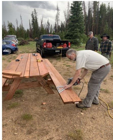
Fred Allen building a picnic table at Stub Creek USFS Administrative Site.
